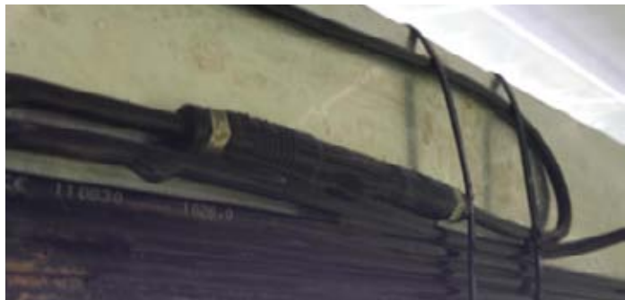
Fig. 9: Fastening of the connector tight to the mounting structure can cause moisture build up between connector and rail, damaging the connection
